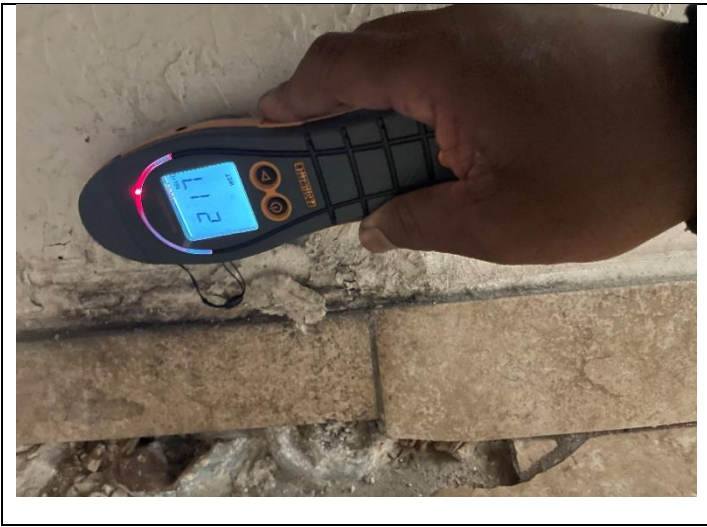
31. View of SVG and elevated moisture using Protimeter under restroom sink in PEI 307
