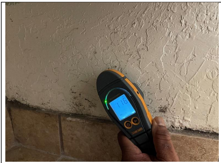
39. View of SVG with dry moisture level with Protimeter under restroom sink in PEI 331
