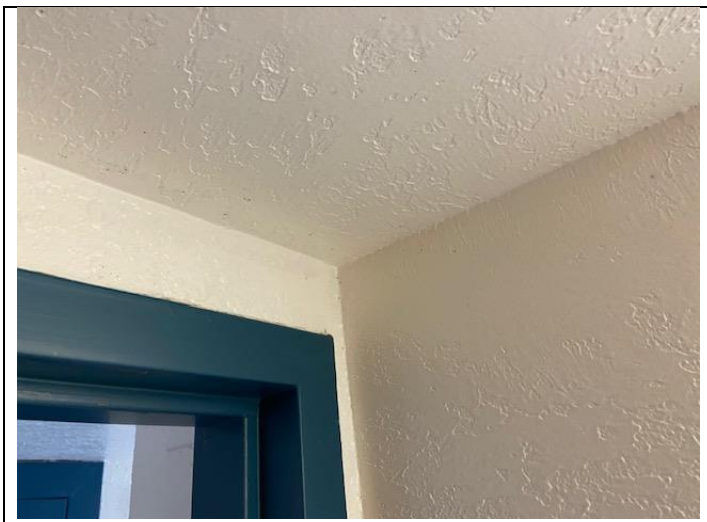
17. View of SVG on unit ceiling (outside restroom) of PEI 232
