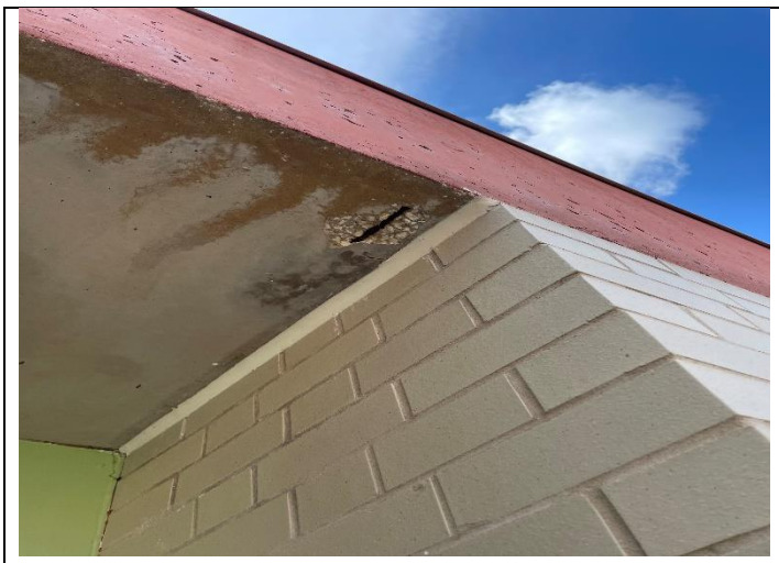
45. View of typical exterior PEI 2 and 3 buildings with visible water damage and spalling of concrete
