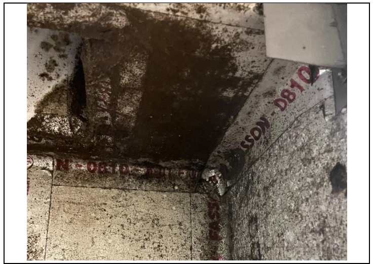
34. View of SVG on top right corner of HVAC system in PEI 315
