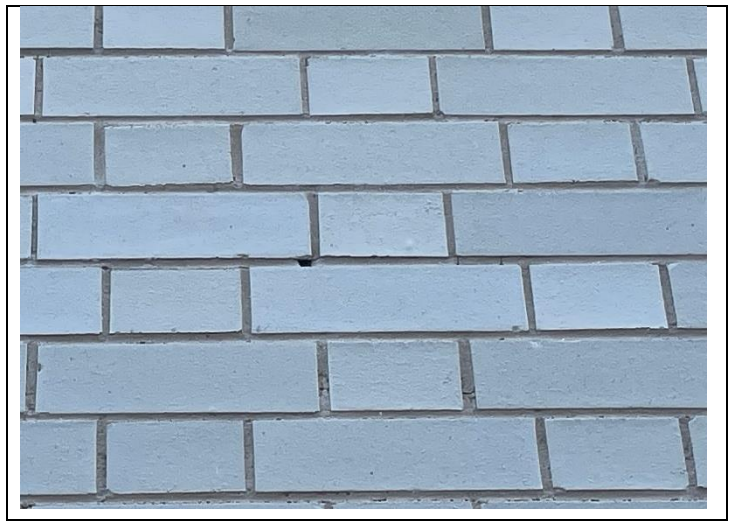
44. View of typical exterior PEI 2 and 3 buildings with identified holes in grout.
