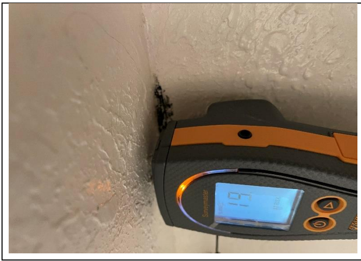
13. View of SVG and elevated moisture levels using Protimeter under restroom sink in PEI 221
