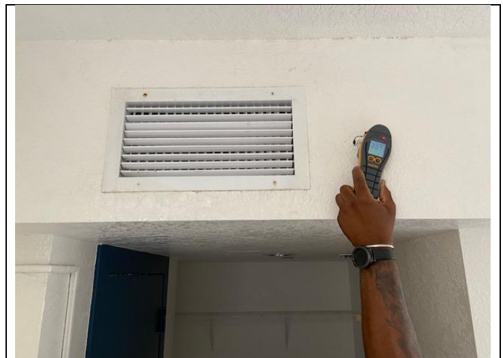
18. View of elevated moisture levels using Protimeter around supply diffuser in PEI 230
