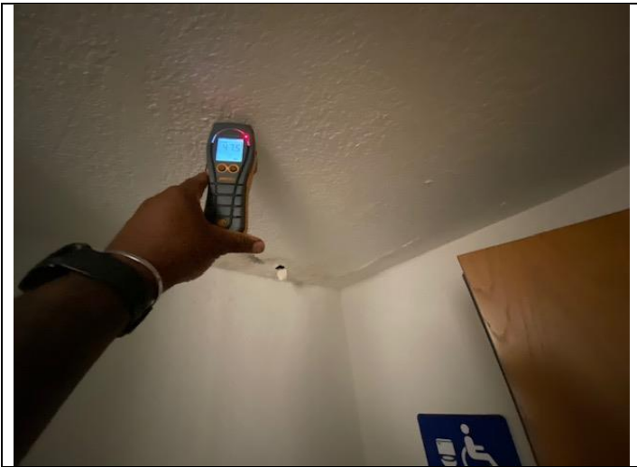
21. View of SVG with elevated moisture levels using a Protimeter on ceiling outside restroom in PEI 2 Lounge
