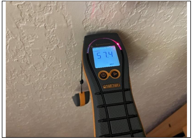
32. View of elevated moisture in ceiling and wall material around HVAC system in PEI 307
