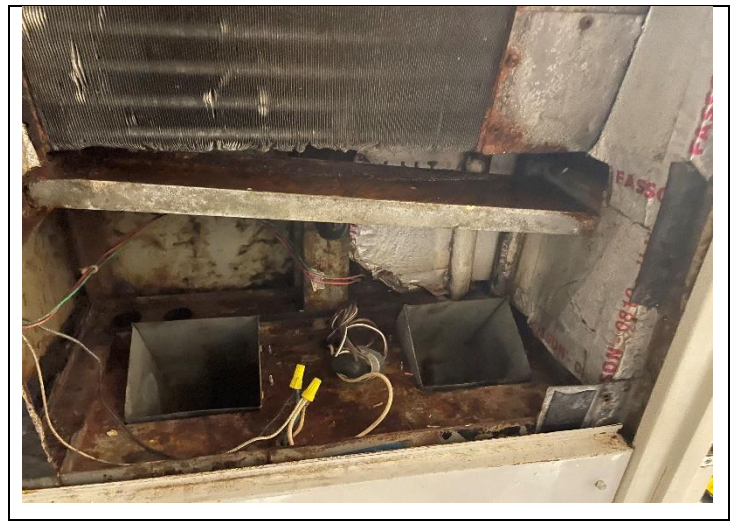
38. View of damaged condensate pan support, draining to wall in PEI 345
