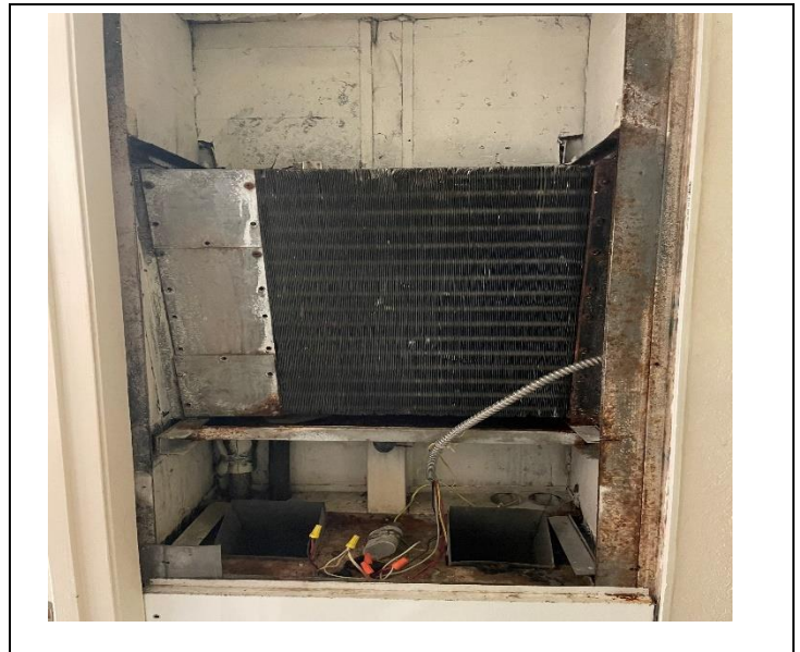
6. Interior view of a typical HVAC unit observed in all units
