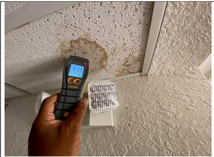
23. View of water damaged ceiling tile with elevated moisture levels using Protimeter in PEI 2 Lounge kitchen
