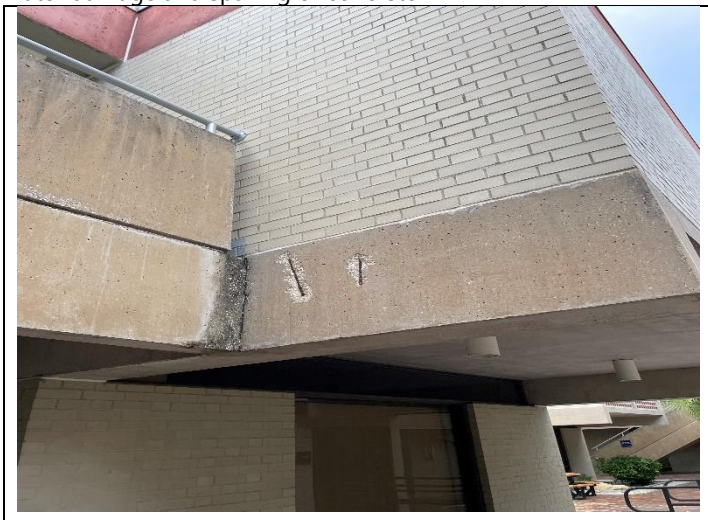
47. View of typical exterior PEI 2 and 3 buildings with visible water damage and spalling of concrete.
