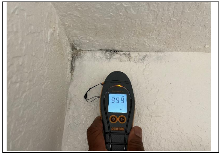
14. View of SVG and elevated moisture levels using Protimeter on restroom ceiling PEI 223
