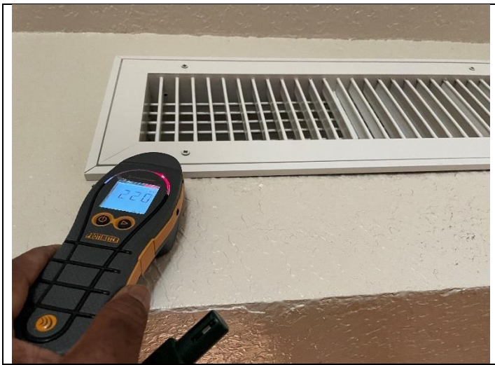
37. View of elevated moisture levels using Protimeter around supply diffuser in PEI 345
