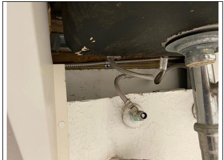
16. View of SVG under sink in PEI 232
