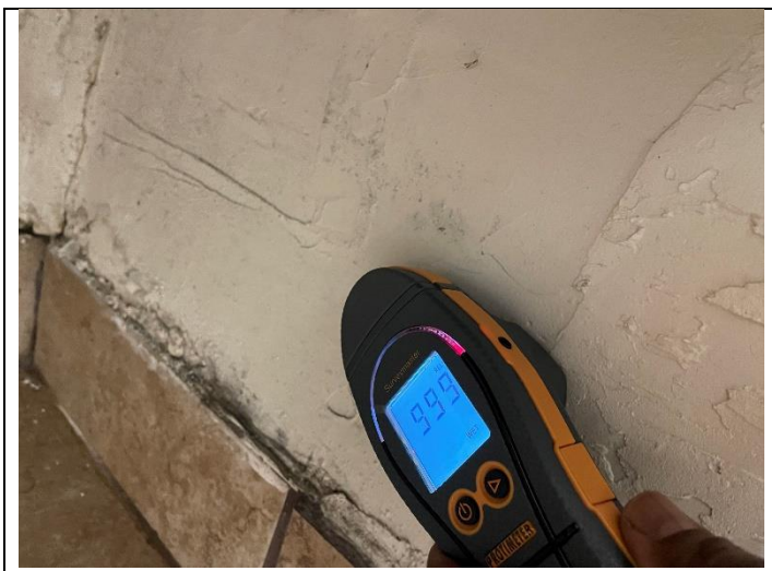
41. View of SVG and elevated moisture level with Protimeter under restroom sink in PEI 308
