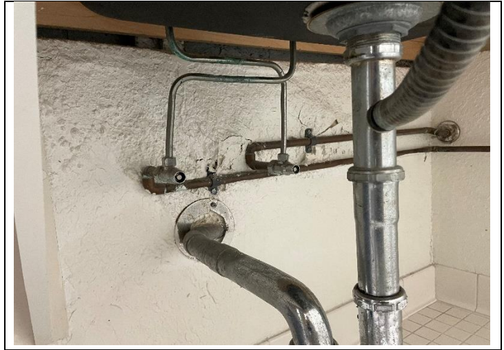
10. View of long term water damage and efflorescence on wall under restroom sink in PEI 205
