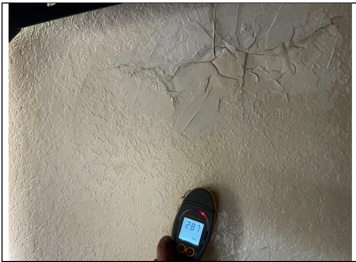
43. View of moisture damage and elevated moisture with Protimeter on North wall in PEI 342
