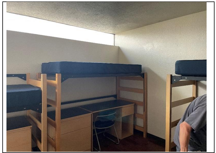
26. View of a typical PEI 3 unit (interior)
