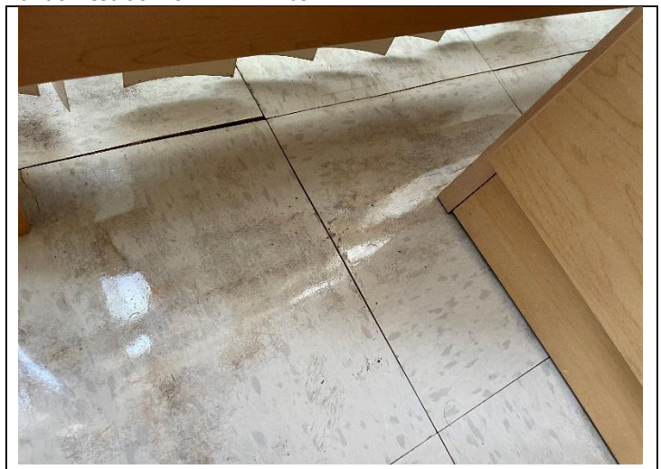
12. View of water-damaged floor tiles adjacent to sliding balcony door in PEI 212
