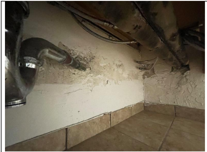
29. View of moisture damage under restroom sink in PEI 305
